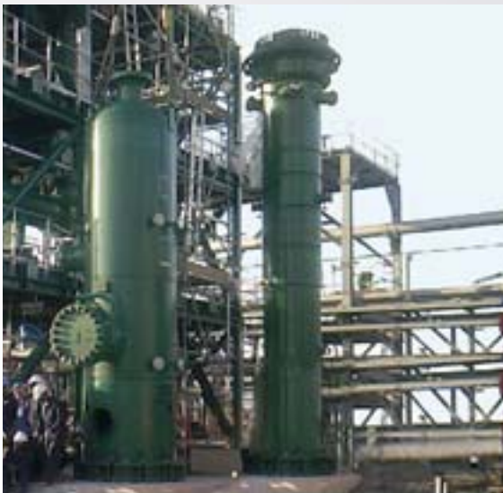
Figure 2 installed Twister Hydrate Separator for JT-LTX system
