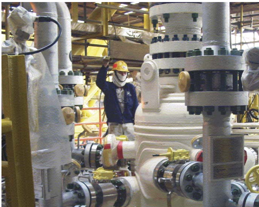
Figure 2. The 300 MMcf/d module on the B11 platform has operated with no downtime for 4 years.
