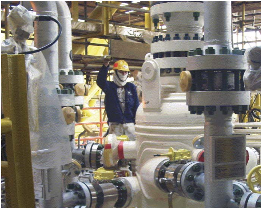
Figure 2. The 300 MMcf/d module on the B11 platform has operated with no downtime for 4 years.
