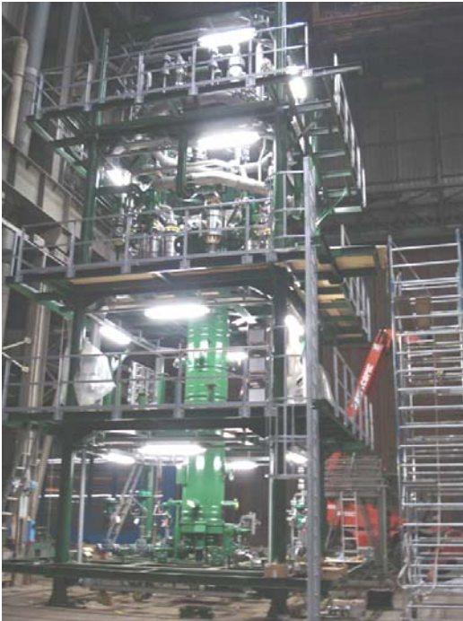
Figure 4 – Twister Gas Processing Module for SPDC Nigeria
