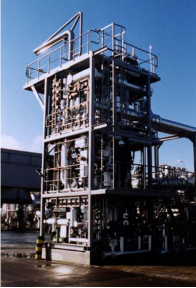
Figure 5 – Twister Gas Processing Module for Petrobras
