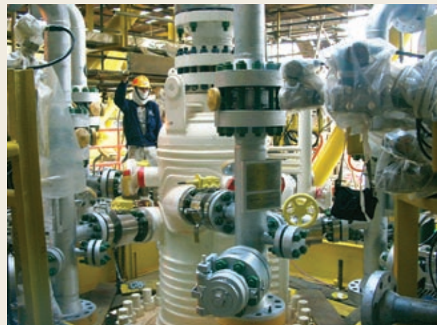
Fig. 4. System in use on the B11 Platform.
