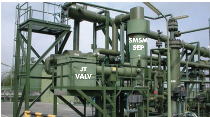
Fig. 2—The LTS train of the NAM Opende Oost gas plant.
