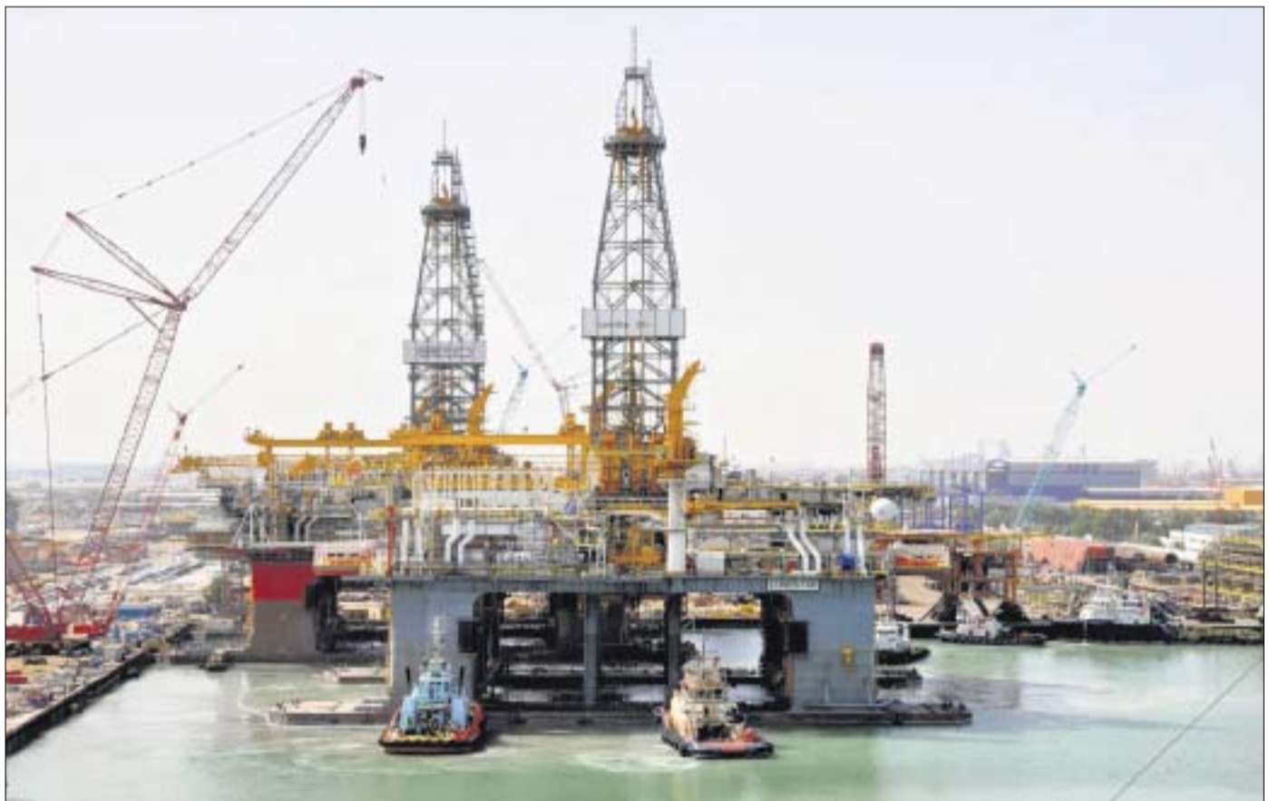
LONESTAR and NORBE VI during construction at GPC yards in Musaffah, Abu Dhabi.
